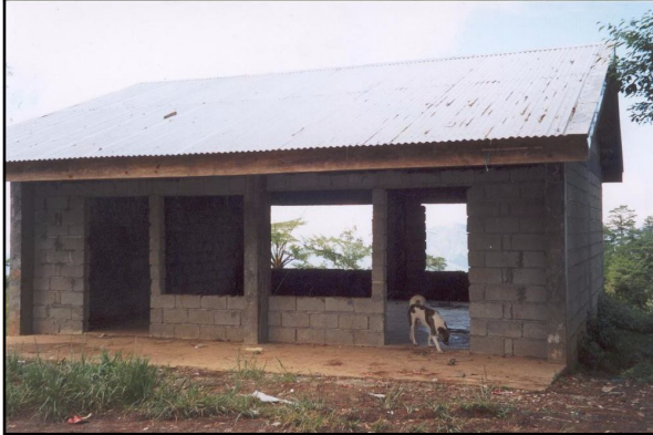
Abandoned School Building (2002) Albis Elementary School, Benguet
